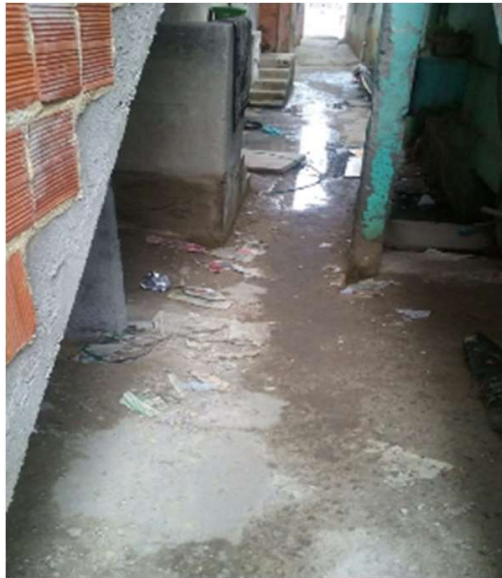
Figure 4-6 – Poor infrastructure of the territory - sewerage
